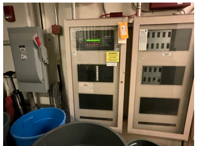
12 - FIRE ALARM PANEL
